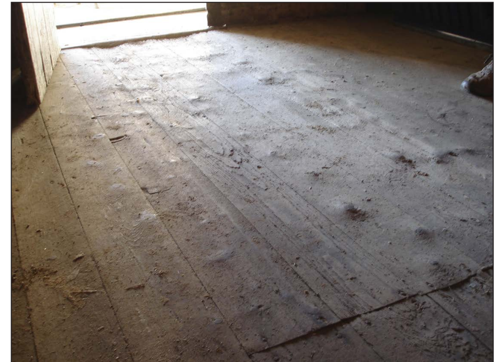
Worn floor boards at door
