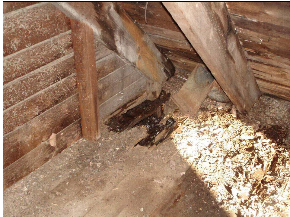
Water damage and rot to roof and floor
